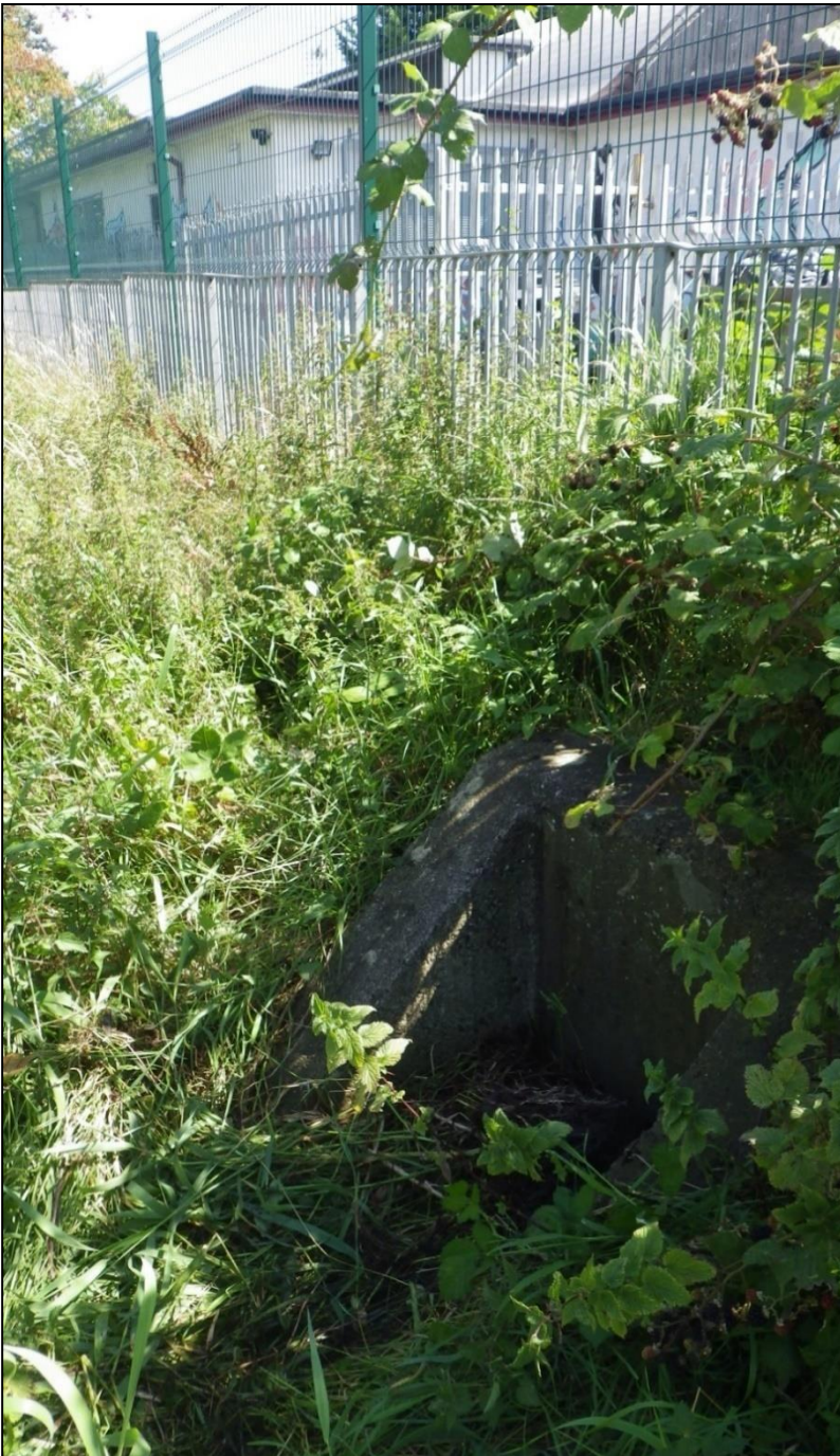
Figure 4: Outfall leading into The Cut, next to the dance studio.
